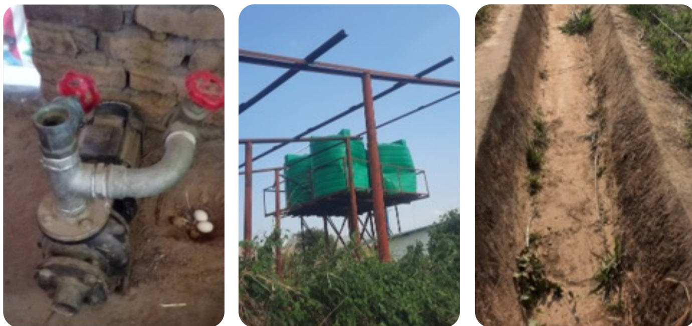
Figure 13: Abandoned water pump, removed solar panels and deformed water tanks and dried canal
